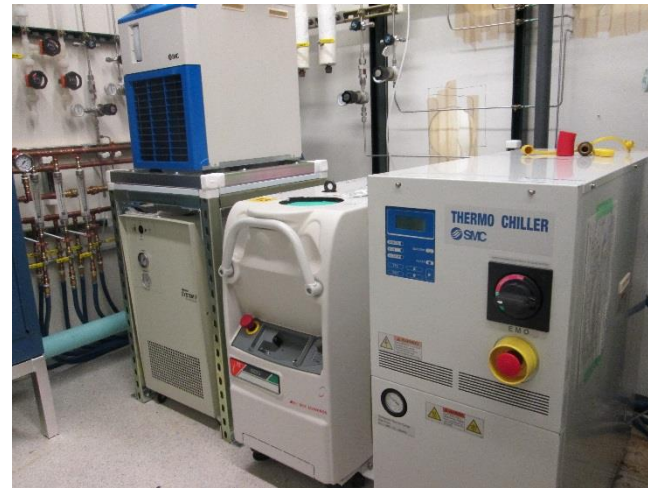
Pump, chillers and heat exchanger in chase
